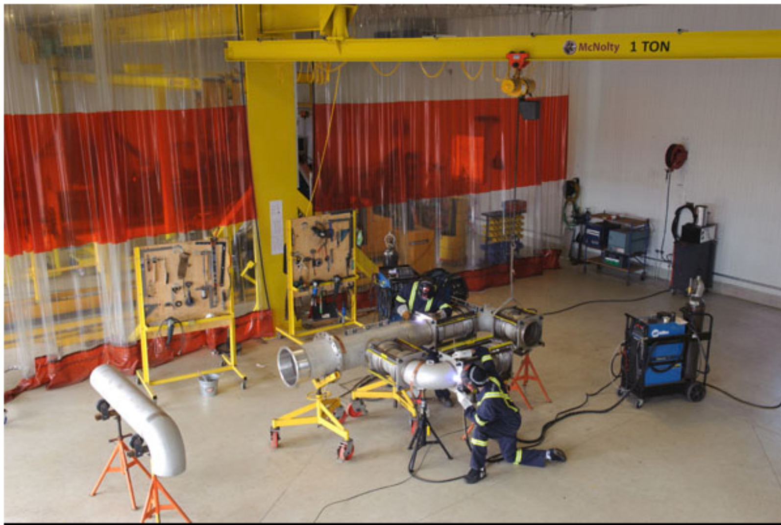
McNolty Mechanical works on a fair amount of specialized equipment, including this high-temperature, 1,800-degree Fahrenheit BLEED AIR piping system for MDS Aero Support Corporation.
